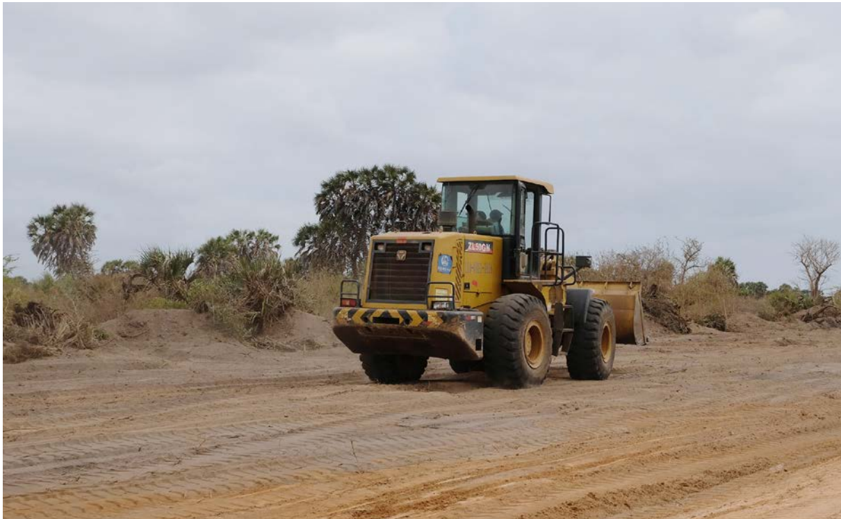
Road construction in the Lamu area has impacted farmers and landowners, who have experienced dumping of waste.
