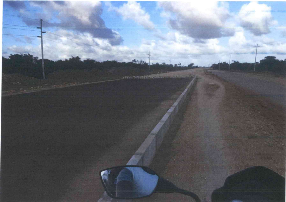
Figure 3: Photo of a portion of the road that has already been tamarked
