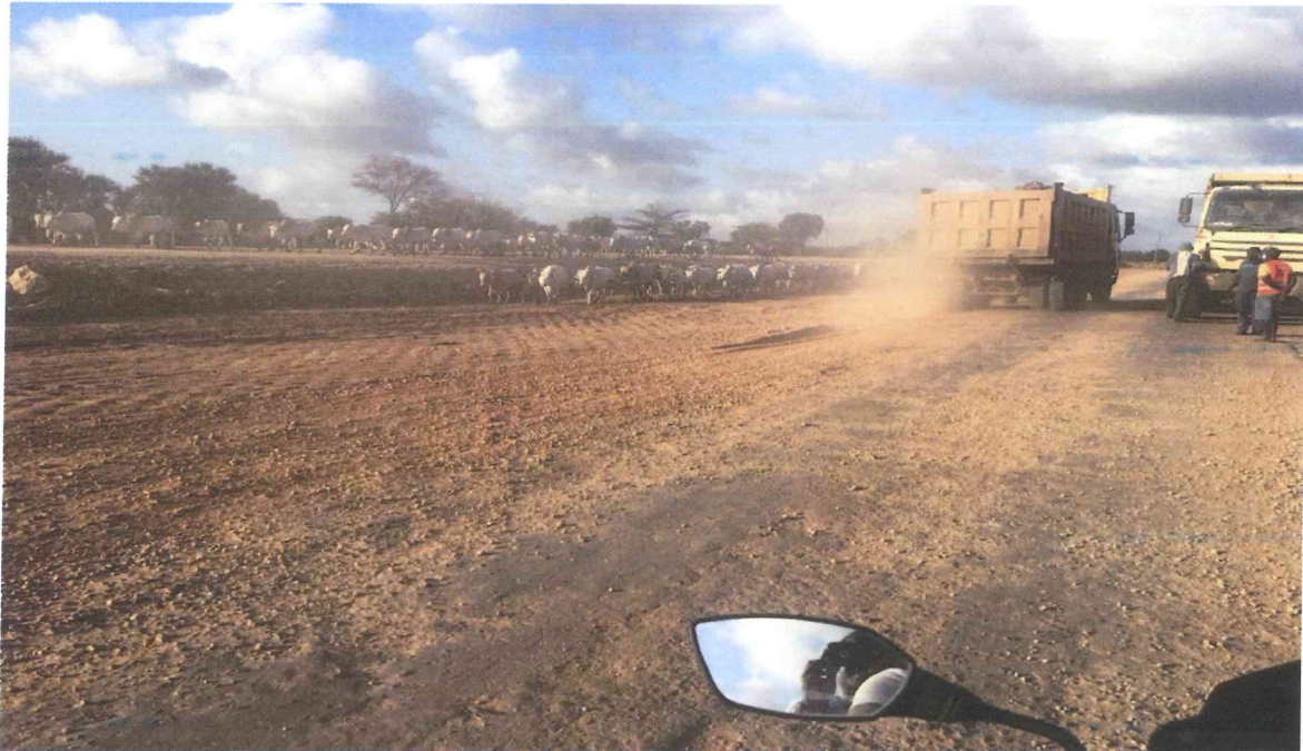
Figure 5: Photo of a tracks transporting construction materials without sprinkling water
