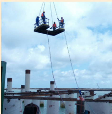
Lamu port construction is well underway with the first berth to be completed in 2019. Natural Justice are assisting the partner organisations to ensure that the construction complies with law.
